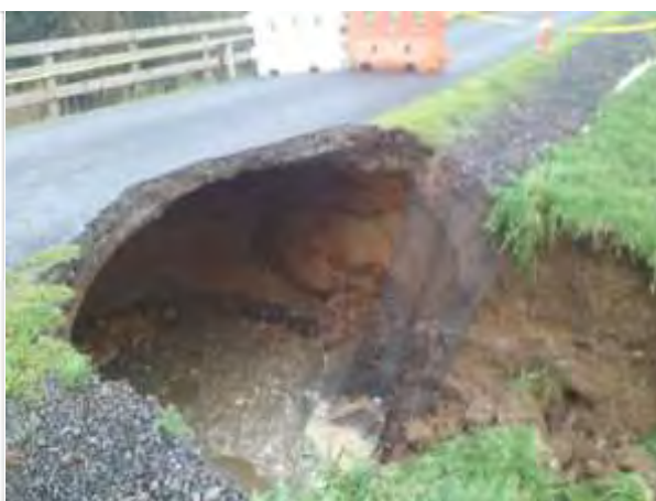
Figure 44 Damage culvert on Nicholson Rd
