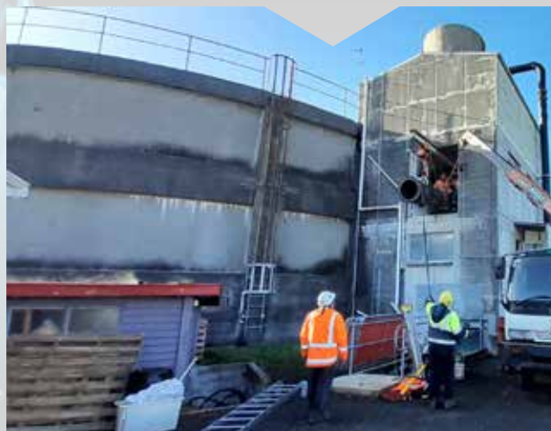
Service Engineers removing the old water pipe that feeds into the Billah Street Reservoir. It was replaced with a new pipe.
