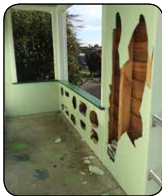
...and the damage done twice over to Council's office in Putāruru cost $1,100 all up.
