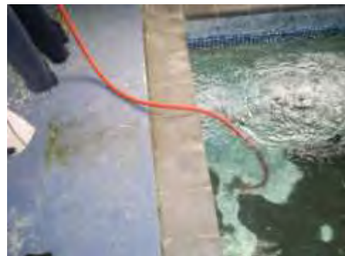
Firehose reel creating a significant hazard to the water supply
