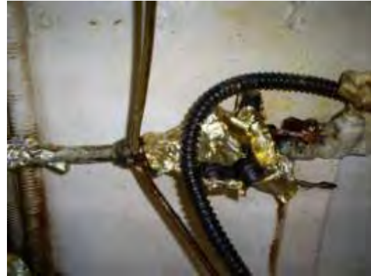
RZP covered in grease - unsatisfactory
