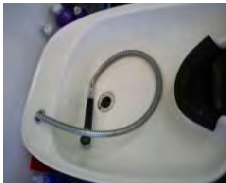
Unprotected flexihose in hairdressers basin
