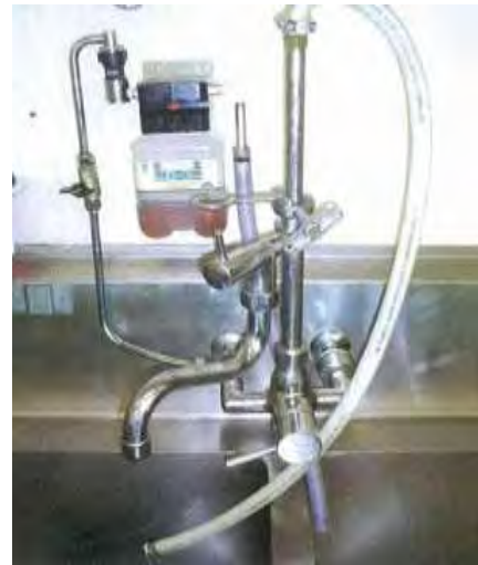
Hazards can exist at outlets intended for food preparation
