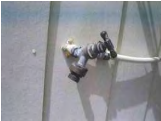
HCVB's require inspection to ensure they are not removed or damaged
