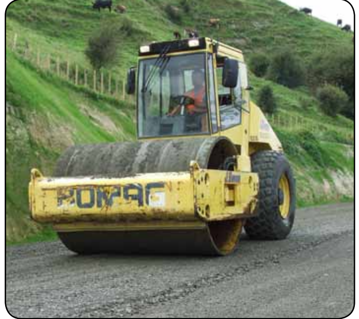
Part of the road rehabilitation process is when the roller compacts the road metal to form a hard surface.
