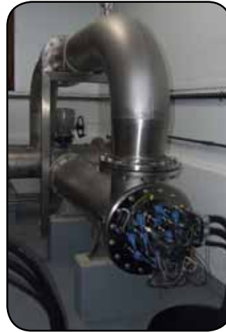
The blue sockets pictured here are connected to UV lights that run the length of the pipe. Water passes over these lights to be disinfected.
