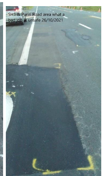
SH1 & Puriri Road area north of Tokoroa one side higher then the other side 26/10/2021 this causes Accident
